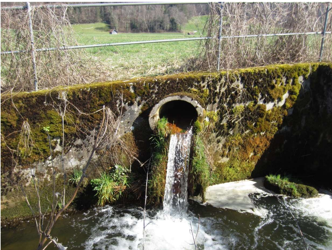
Figure 3: A drain probably discharging more water than just drained water.
